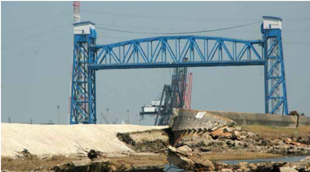
Figure 1. Failed flood wall near the Florida Avenue Bridge. (Photo courtesy of U.S. Army Corps of Engineers.)
