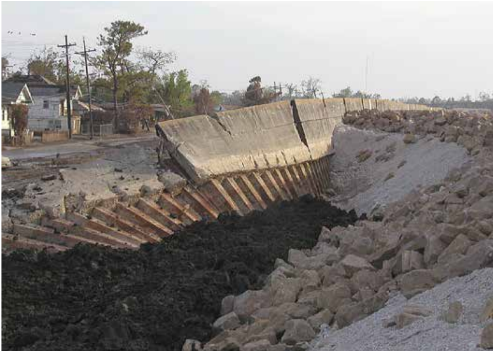
Figure 3. Rotated I-wall. (Photo courtesy of USACE.)
