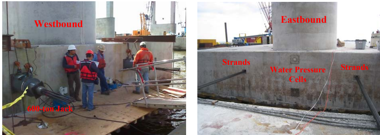
(a) Jacking System at the Live-End of Westbound Pier (b) Eastbound Pier with Steel Strand Tendons
